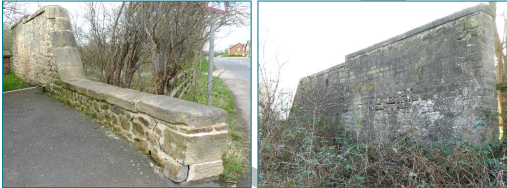
Remains of southern boundary wall of the original [D] Coal Depot constructed in squared sandstone. Left: Viewed looking north with Sadberge Road to the right. Right: Viewed from the railway corridor looking south. (Photos © Gaby Rose, March 2024)
