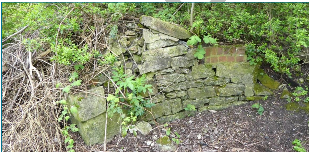
Top: Remains of [G] Enclosed Railway Corridor in Pease brick laid in an English Garden Wall bond (like the [C] Waiting Shed) to the north of the former Gas Works and windmill sites; note the 'zigzag' line of wall (Photo © Gaby Rose, March 2024). Middle: Remains of later, southern coal drop walling of the [D] Coal Depot built in stone; the brick walling on top was added when the depot was no longer in use. The wall now forms the boundary to the carpark of the former [E] Fighting Cocks Inn. Bottom: This feature, judging from its position near the [A] Crane Base and Platform (just outside this view on the right) and on the 1913 map (see below), seems to be related to the ramp carrying the siding track to the coal cells. (Photos © Gaby Rose, April 2024)
