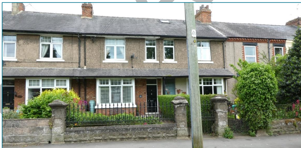
Subzone D1: Top left : Stone-built terrace of c.1900 with canopies spanning between bay windows with shallow front garden. Whilst the window frames have been changed to different designs, this terrace is otherwise well preserved. Top right : Entrance pier with carved stone cockerel and commemoration plaques on gable in the background, [J] Cocks Memorial Homes. Middle : The long Station Terrace with three well preserved houses, although window frames have been changed to different designs. The unit on the left, which would have looked the same, has been changed significantly. Bottom : Water View, the southern terrace, of which parts have been rendered. Note the eaves detailing on the right-hand house. Again, there is a ground-floor canopy and the original opening pattern has been preserved. The front garden has an unusual stone boundary wall with metal railings and distinct carved piers, which are in poor condition. (Photos © Gaby Rose, May 2024)
